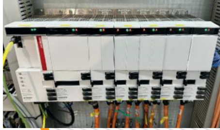
08 Reliable Beckhoff CNC Controls
